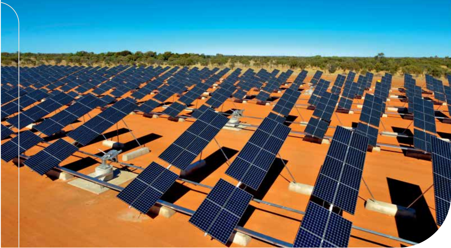
Above: Uterne Solar Power Station, Alice Springs.
