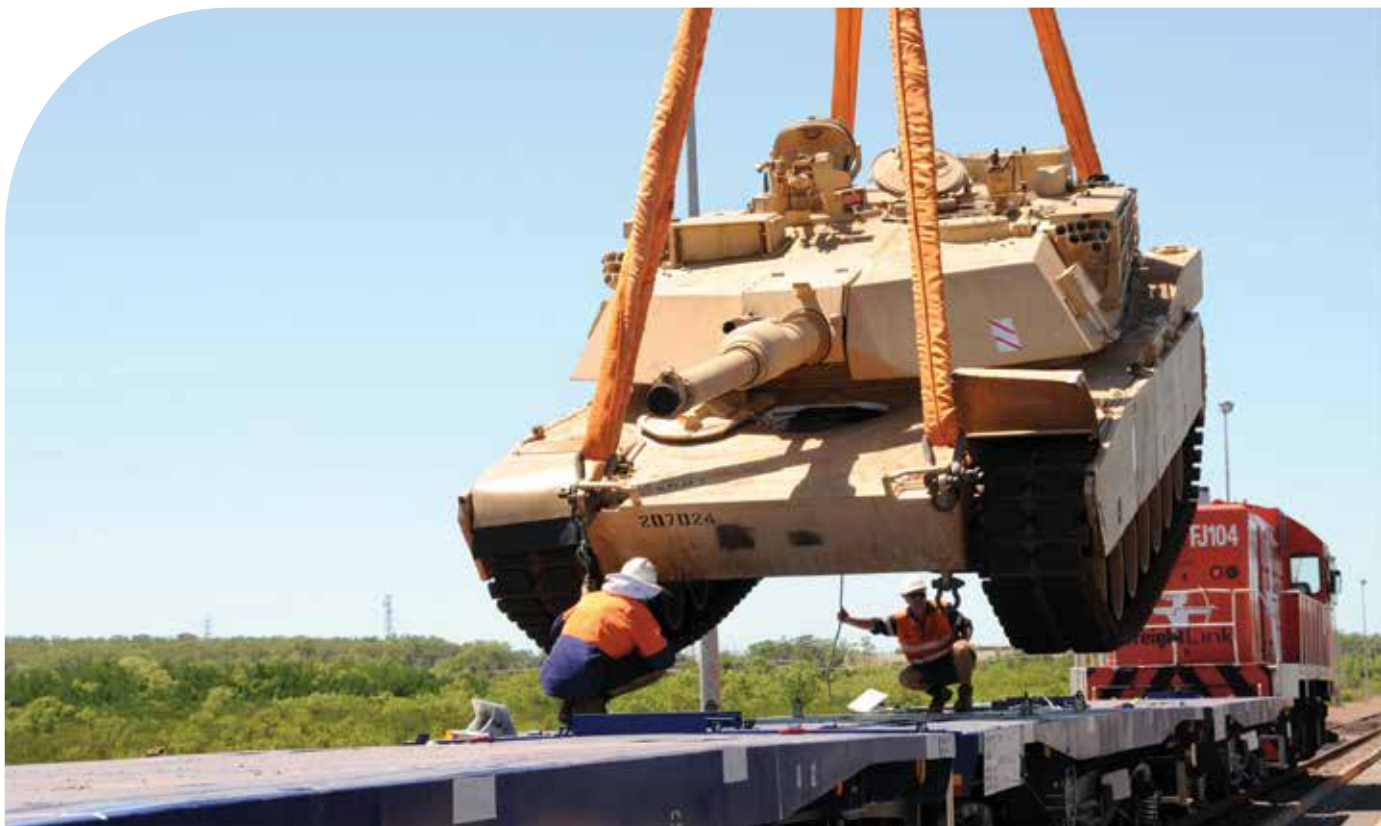
Above: 60,000 kilograms of armour touches down onto the purpose-built rolling stock during loading trials. Credit: Department of Defence. © Commonwealth of Australia, Department of Defence.
