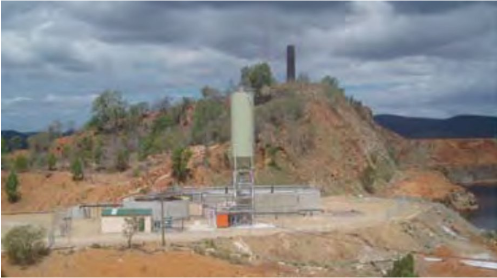
Figure 5.21 - Pit water treatment plant adjacent to the AMD-filled open pit at Mt Morgan (March 2006).
