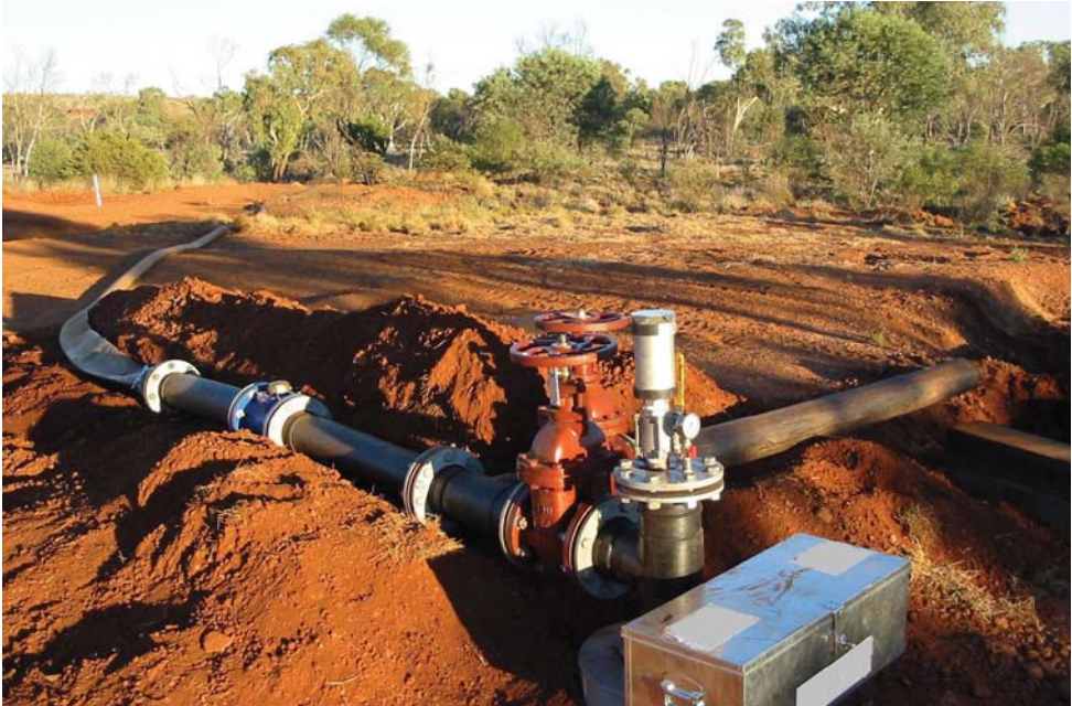
Figure 4.24 - Mine dewatering water re-injection at Yandicoogina
