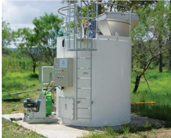
Figure 31: Generator-powered portable mixing and dosing system for remote sites
