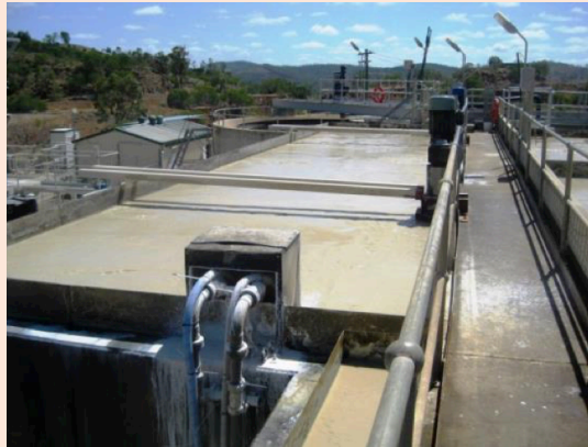
Figure 1: Mount Morgan mine lime-dosing water treatment plant—neutralisation tanks
