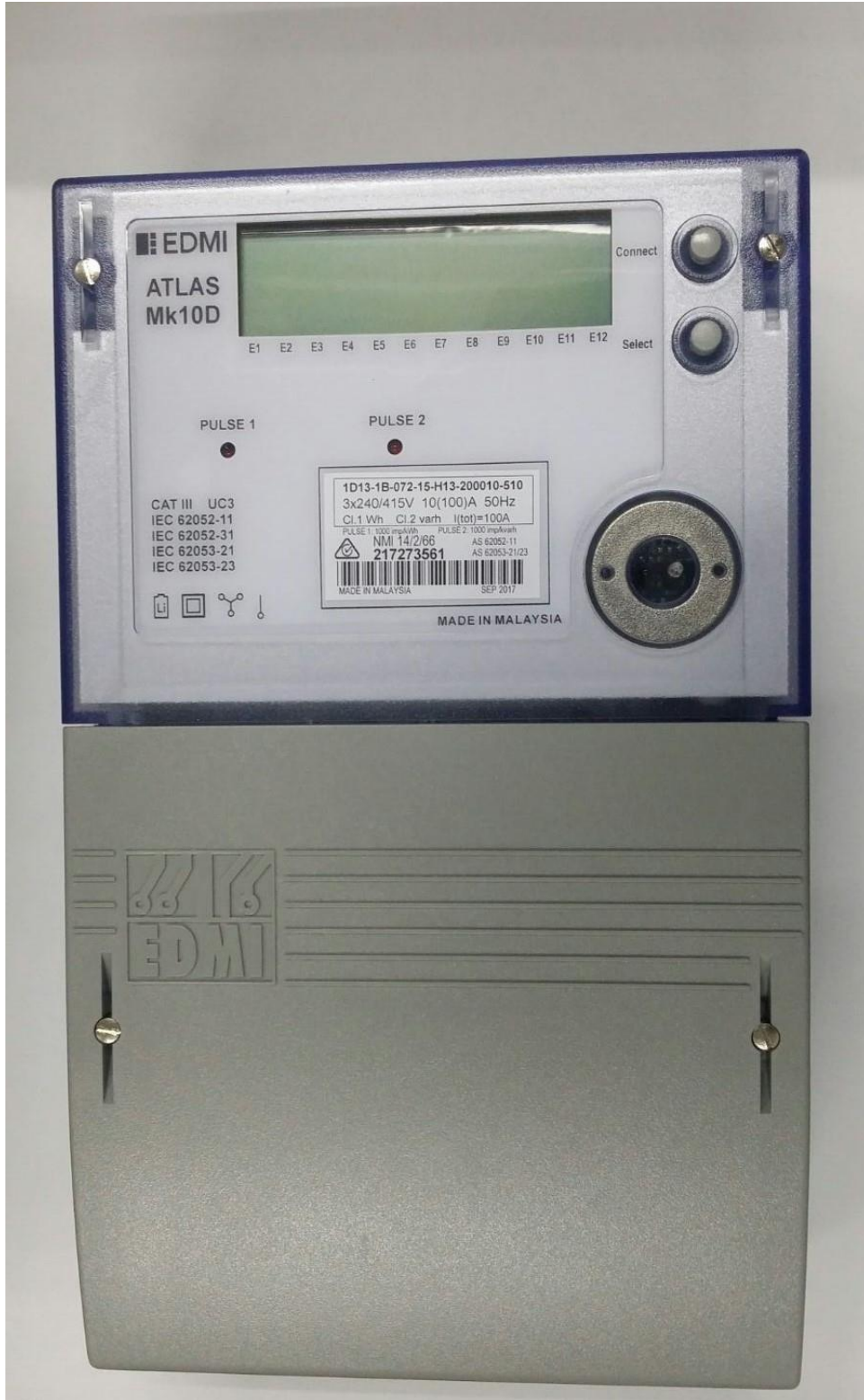
Variant 1 of EDM I Model Mk10D Class 1 Electricity Meter (Including Typical Mechanical Sealing)
