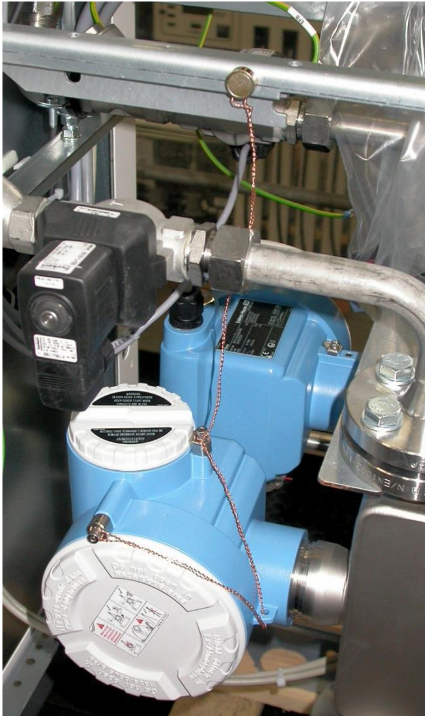
Typical Sealing of Coriolis Meter Calibration Access Including ModBus Connections (Variant 22)
