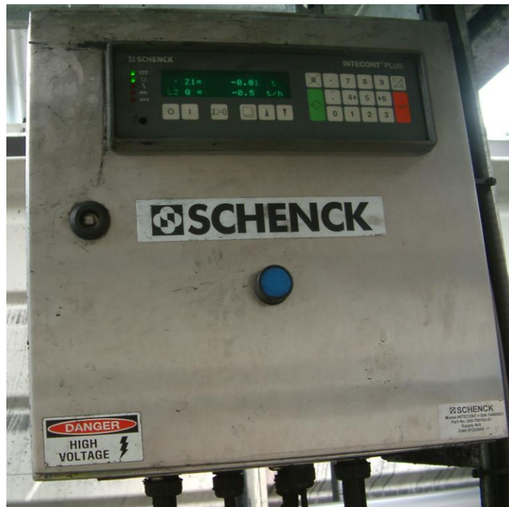
(b) Intecont Plus Indicator in Additional Housing
