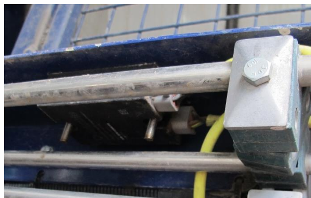
(c) Angle Sensor Located to Detect Out-of-Level Conditions
