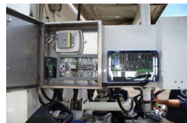
Typical Banlaw FuelTrack Installation
