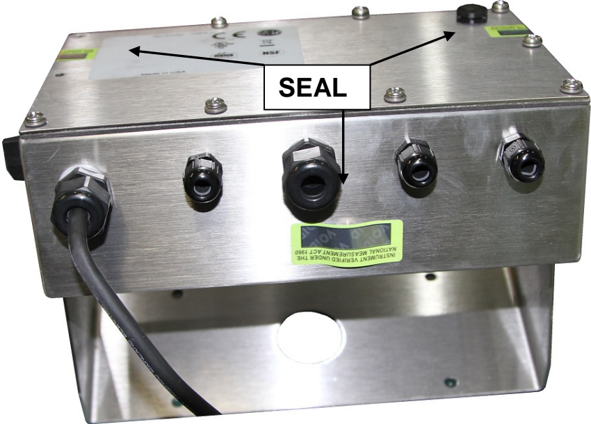
(b) Typical Sealing Using Destructible Adhesive Labels
